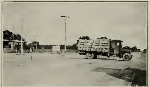
—Courtesy Pacific Portland Cement Co. Pavement open for traffic at 9 A. M., April 11, 1932. Cores tested on the afternoon of April 10—24 hours after being laid—showed a compression strength of over 2000 pounds per square inch. Six-sack mix was used.
